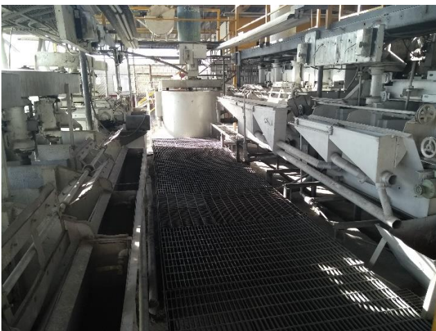
Photo 3: The lead float zinc reconditioning and reagent mixing area with the lead float to the right.
