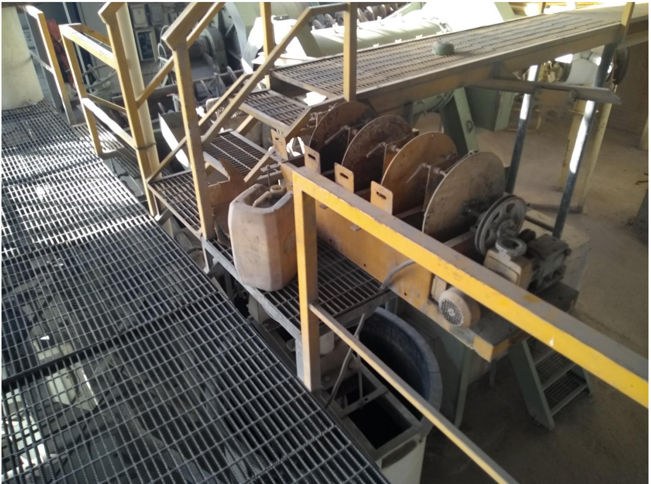
Photo 7: Lead preconditioning tank in the foreground with the reagent dosing facility sitting above the lead preconditioning tank
