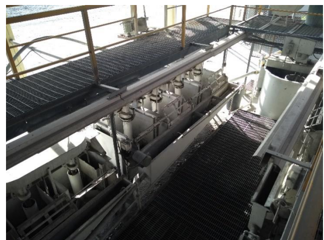
Photo 4: The zinc float and process control walkway
