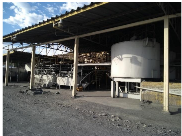
Photo 2: Zinc float cells, lead thickener and drying bunkers in the right background.
